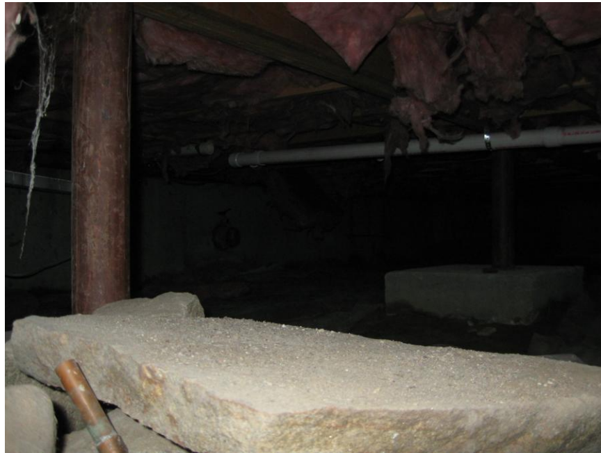
The crawlspace needs rubber sheeting applied to it to seal it from water.
