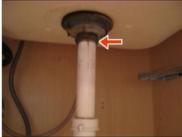
4.0 Picture 1 Right sink basin
