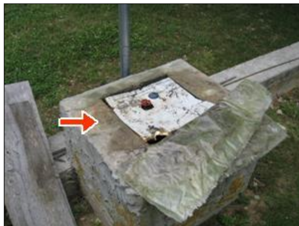
4.1 Picture 3 Well head
