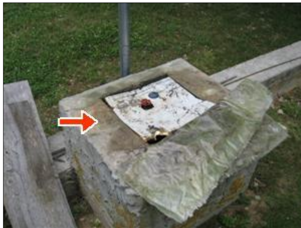
4.1 Picture 3 Well head
