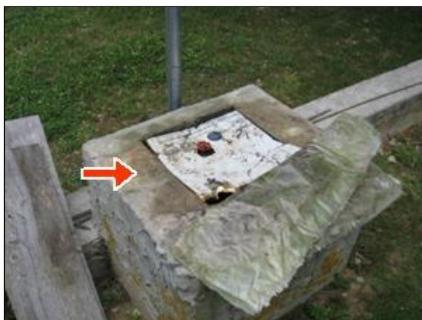
4.1 Picture 3 Well head
