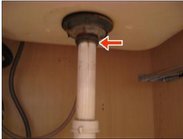
4.0 Picture 1 Right sink basin
